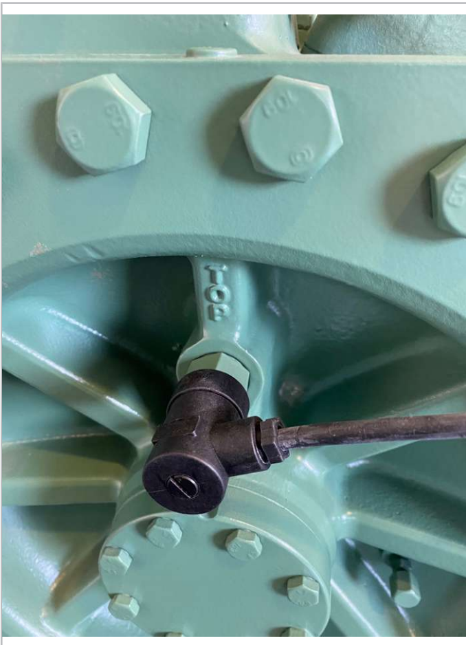
Fig. 40: Differential oil pressure switch DP-1 at the compressor (example)
