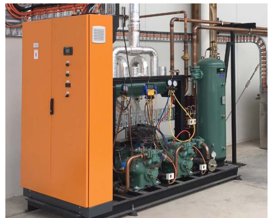
Twin compressor rack
